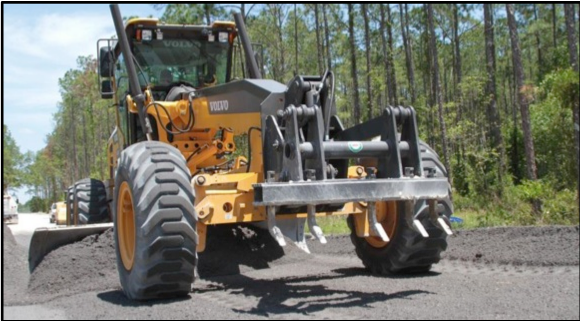
Figure 3. WTE ash road base course being placed by Pasco County Road and Bridge
